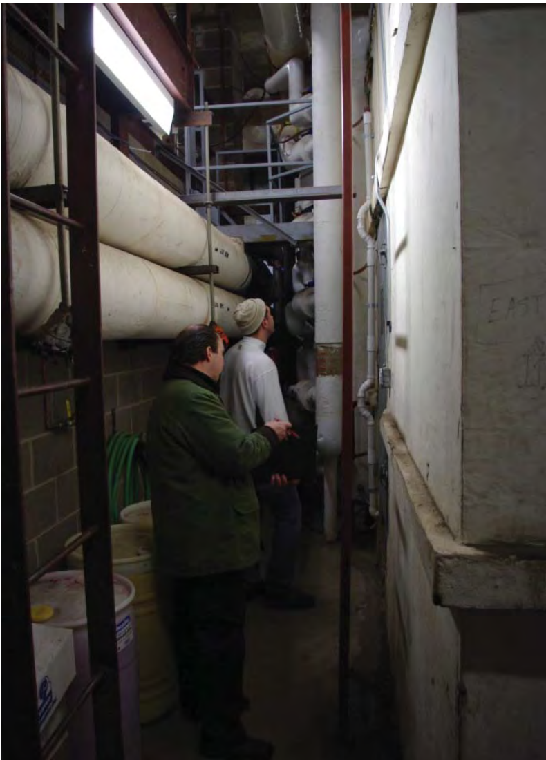
DANIELS MECHANICAL ROOM - 9TH FLOOR
